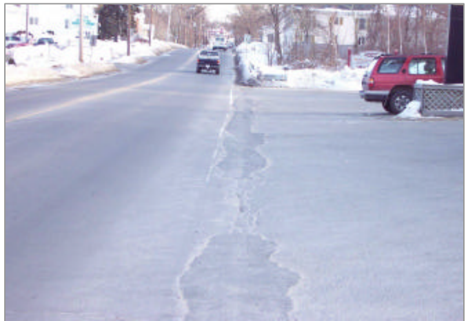
An example of a “lot wide” curb cut on Route 38 in Tewksbury. Photo by Wayne Darragh, March 2003.
